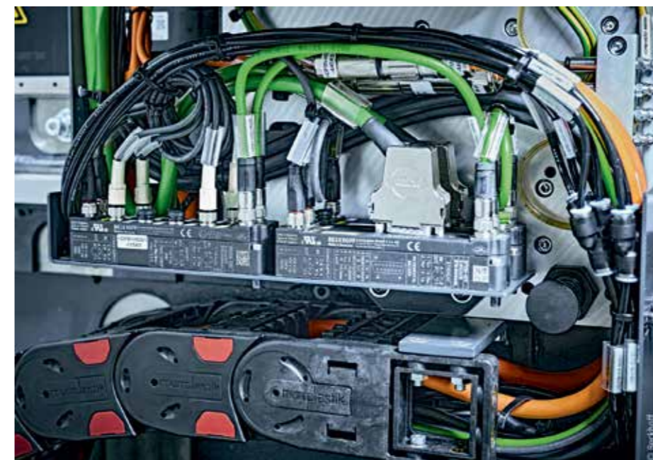
The wide I/O spectrum of IP20 EtherCAT Terminals and IP67 EtherCAT Box modules (here: EP2338 and EP5101 in the BLS 500) facilitates the modularisation of Manz systems.
